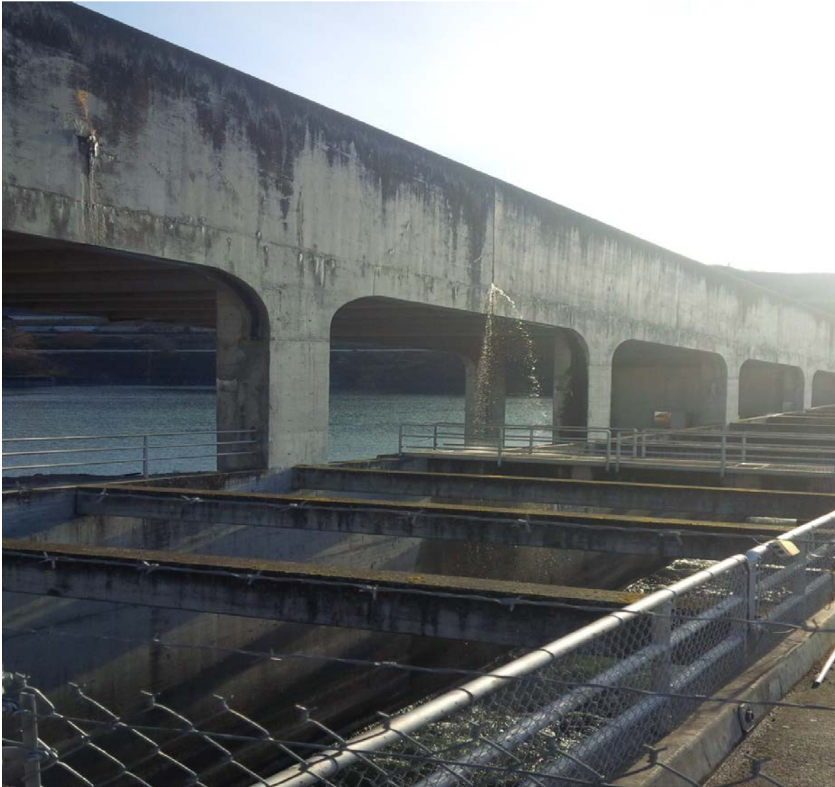
Leakage increase from east ladder expansion joint with decreasing temperatures.
